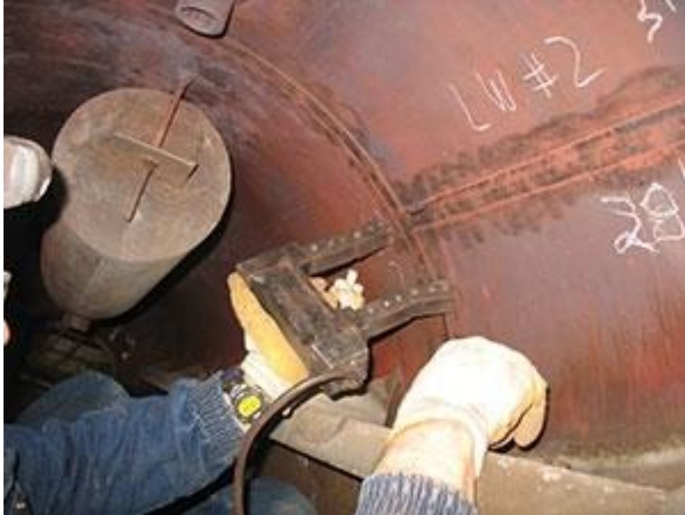
Use of an AC yoke in the MT process to detect fatigue-type discontinuities in welded seams of a steam drum during inservice evaluation.
