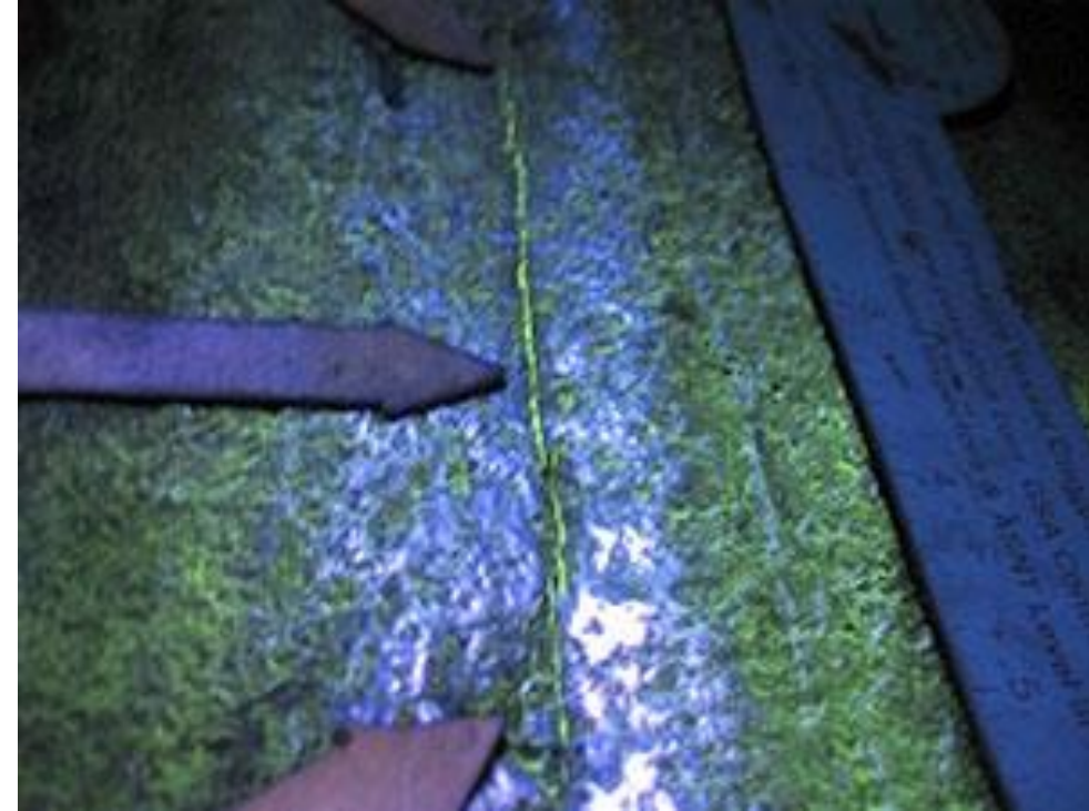
Wet fluorescent MT process showing a crack in a steam drum circumferential weld seam.
