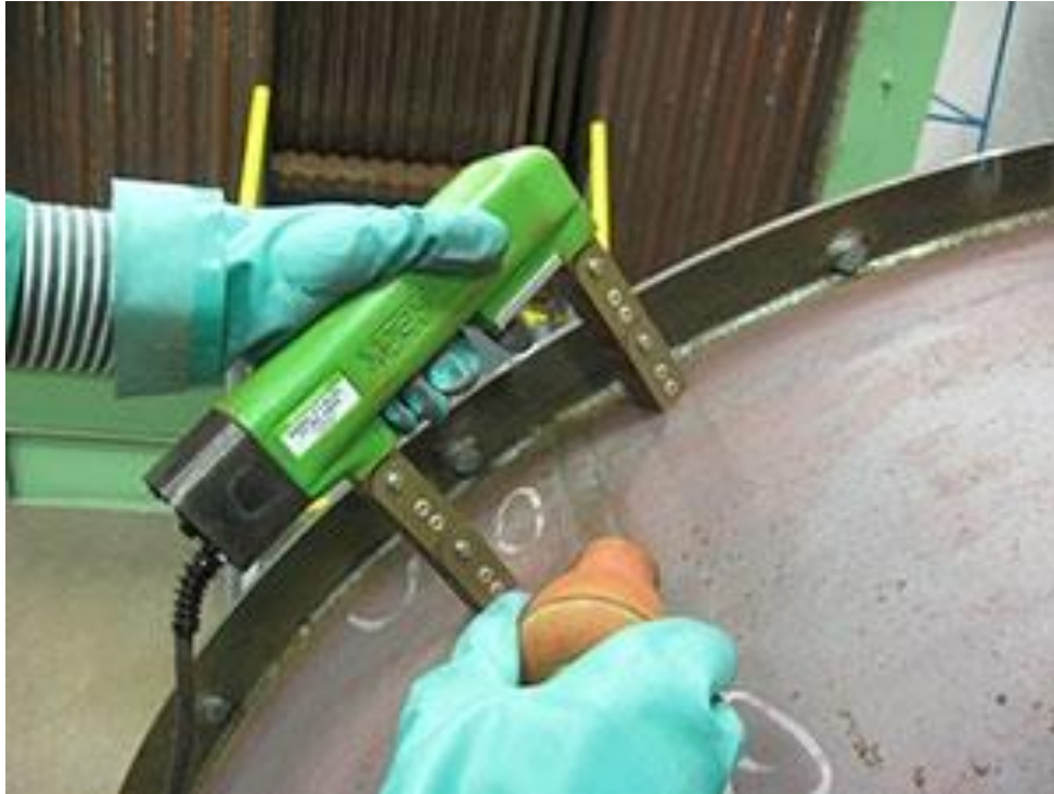
MT examination of the longitudinal seam on an inservice boiler.
